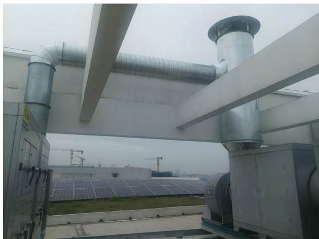
Waste Gas Treatment Equipment
